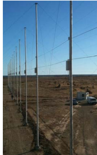
Figure 10(c) – Matching filters installed on site
